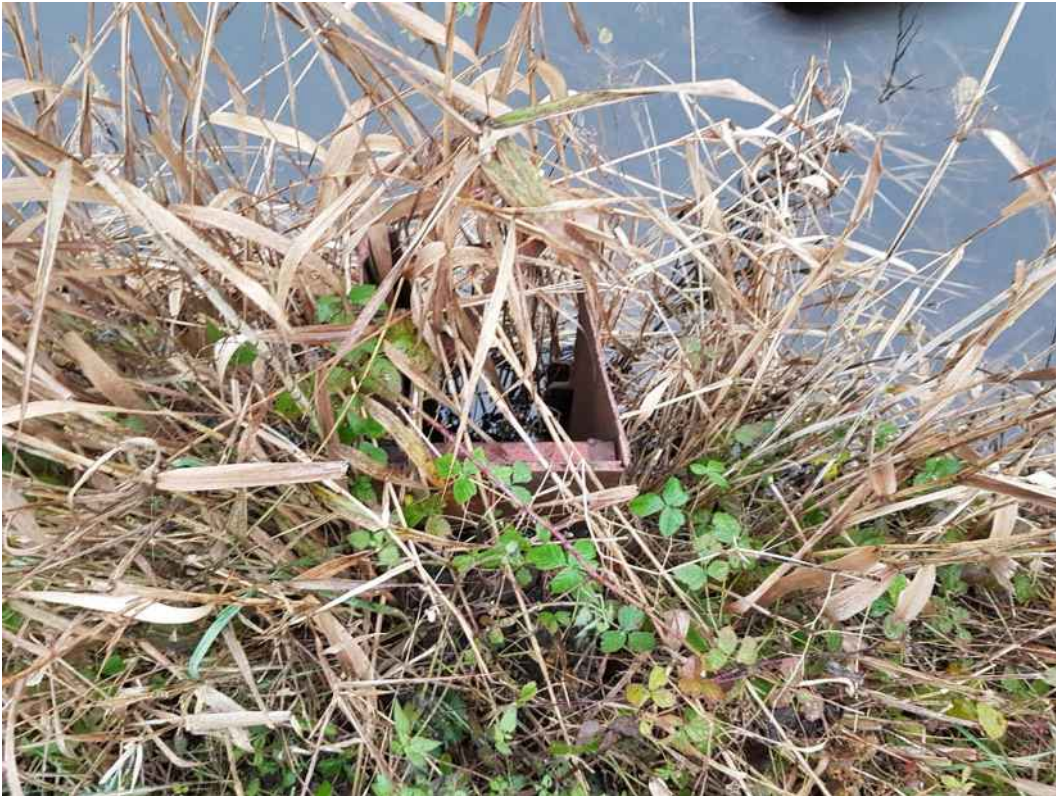
Photo B.6: Control structure with one-way valve on Black Ditch
